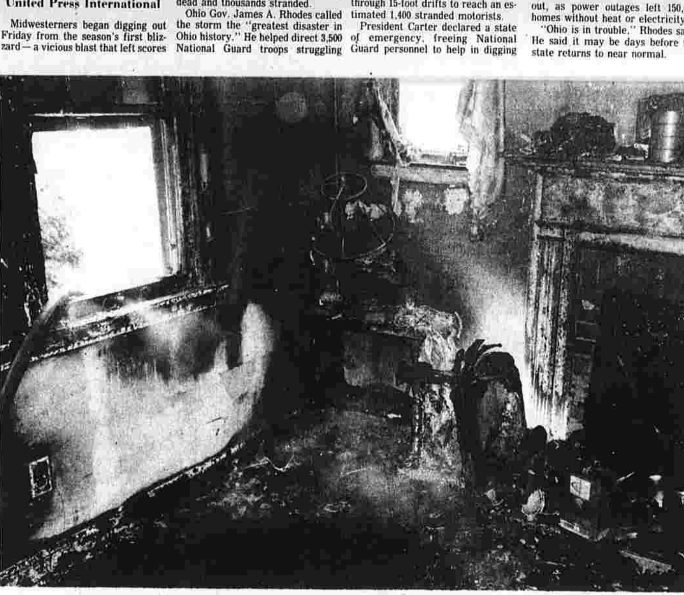
The living room of this home at 29 Whitney Road was extensively damaged by fire Friday afternoon. A fireman and an occupant of the home were treated for injuries. Three cans of gasoline containers were at the base of the fireplace, but did not explode in the fire. The Town Fire Department had not determined the cause of the fire. (Herald photo by Pinto)
